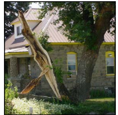
This tree split out where multiple tops converged from one spot. Early pruning to establish a single trunk and good branch structure could have prevented this damage.
